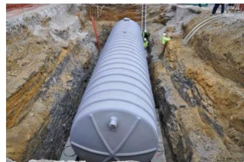
Figure 14: Underground storage tank. (Source: Vergroesen et al., 2013)
