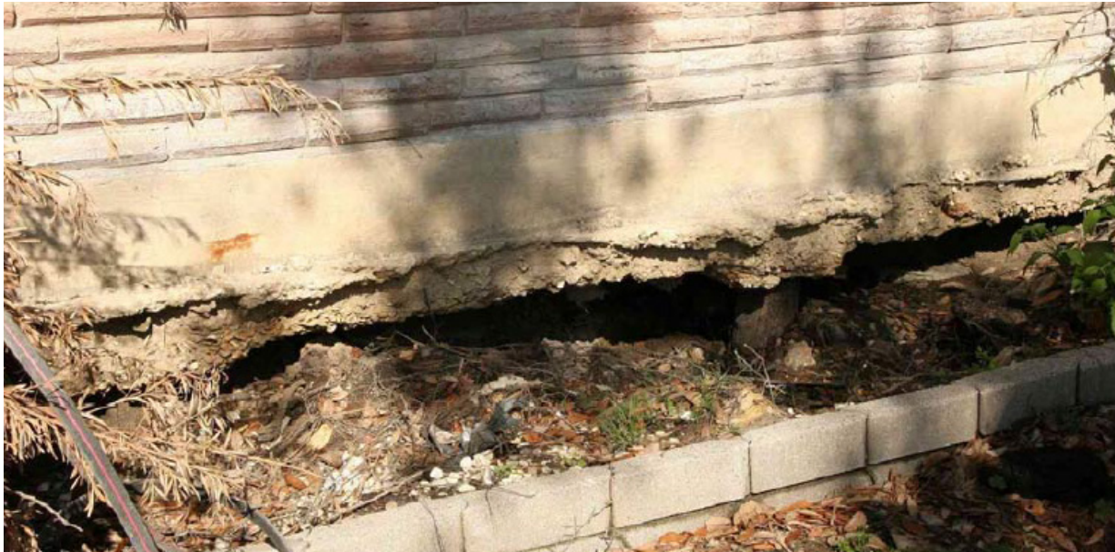
Figure 3.22 Ground settlement/subsidence relative to a house in lower New Orleans. From: ILIT (2006)
