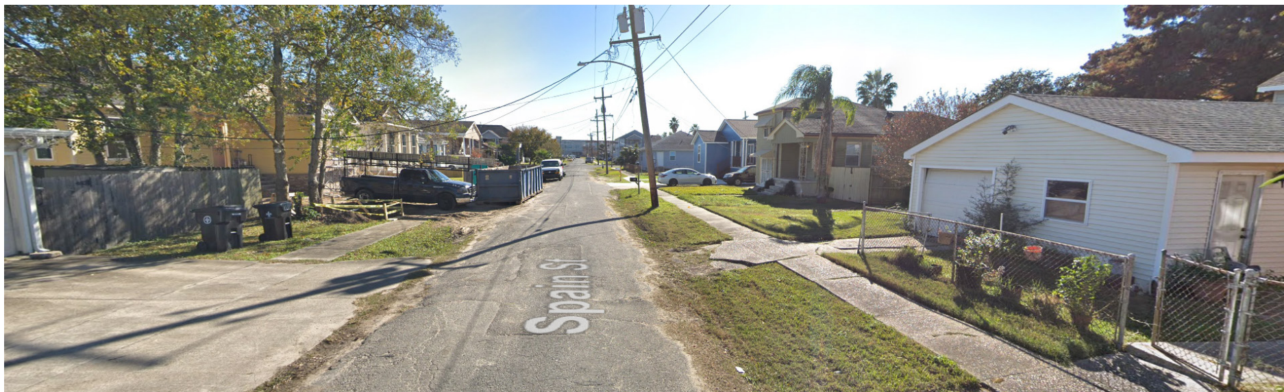
Image 9.1. Pavement in poor condition in Gentilly District. Source Google Street View, retrieved March 26, 2019
