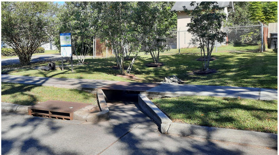
Figure 6.13: Example of a catch basin next to bioswale inlet. (source: https://www.climatescan.org/projects/9695/detail )
