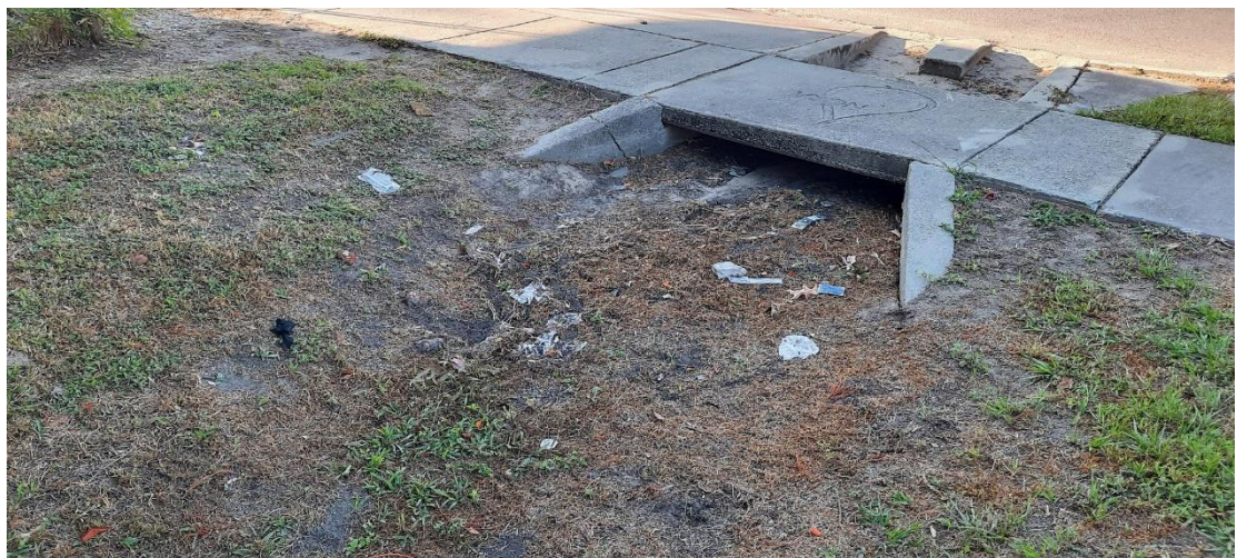
Figure 6.12: sedimentation and (visible) pollutants at bioswale inlet. (source: https://www.climatescan.org/projects/9685/detail )
