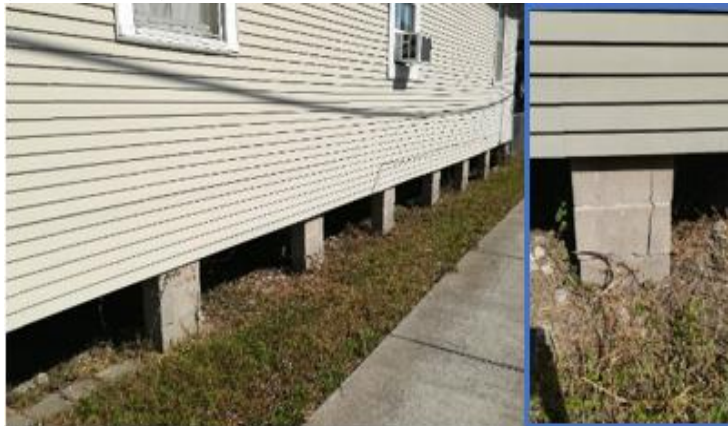
Figure 6.1.1: Cracks in foundation (N Rendon St/ Bienville St; Bayou St. John)
