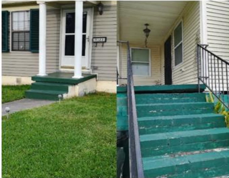
Figure 6.1.3: subsidence of front door stairs (St. Anthony)
