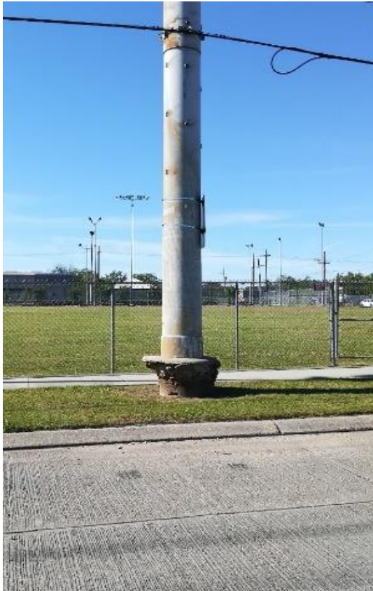
6.2.5: Indication of land subsidence (New Orleans)
