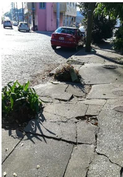
Figure 6.2.1 Cracking road (Lower Garden District'; Felicity St/ Richard St)
