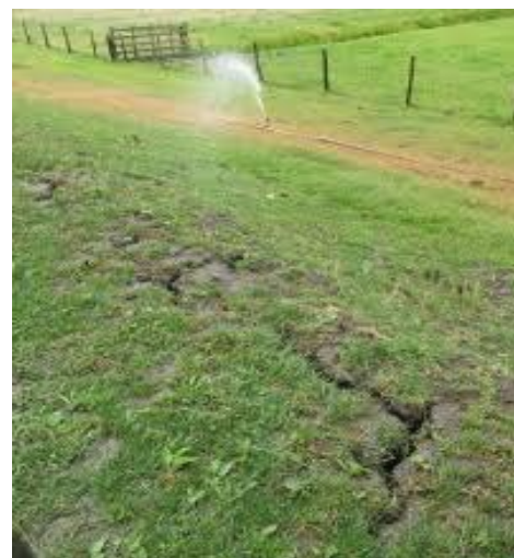
Figure 5.3.2: Cracks due to dehydrated soil. Source: (Deltares, 2018c)
