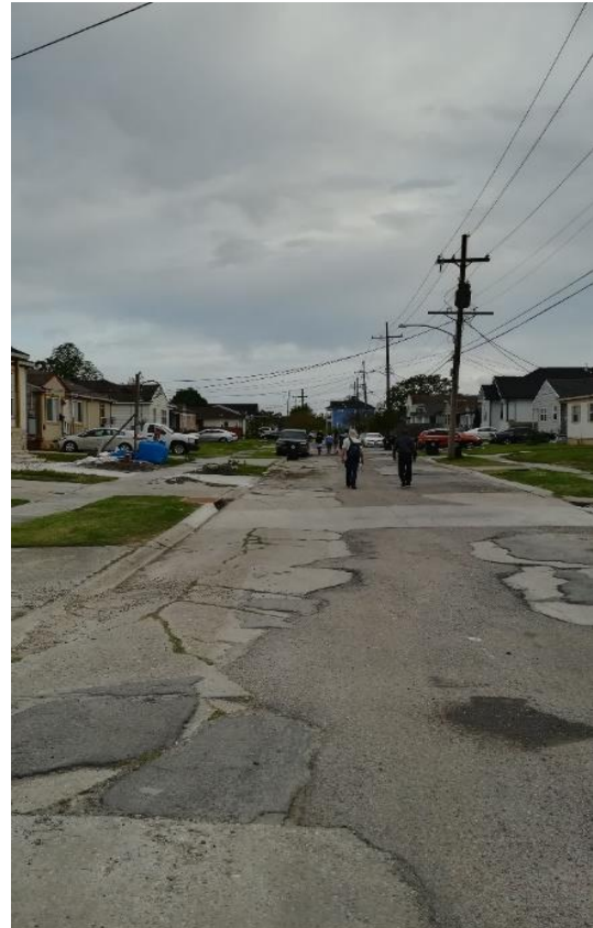
Figure: 6.2.6: Overview of a road which has partly subside and partly repaired (St. Anthony, Warrinton Dr)
