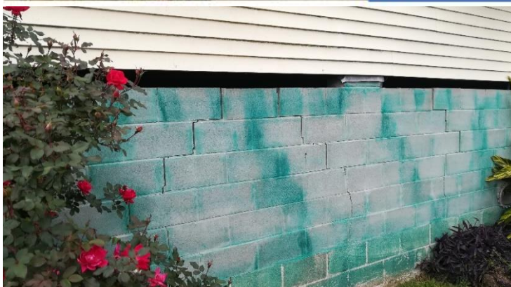
Figure 6.1.2: Cracks in walls (St. Anthony)
