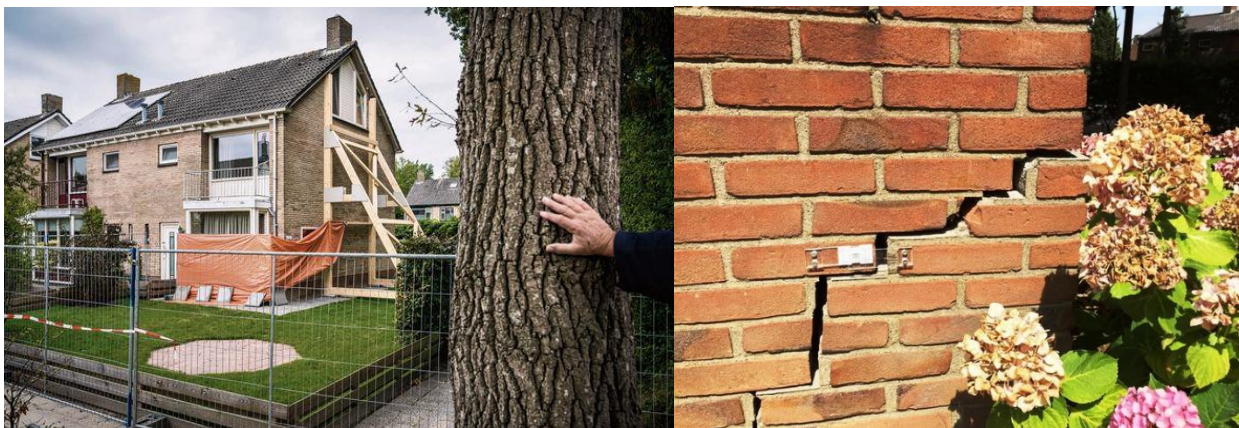
Figure 5.2.2: As a result of land subsidence, two houses have been stabilized to prevent collapsing. Source: (Schreuder, 2018)
