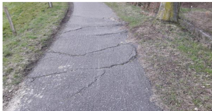
Figure 5.1.2: tree roots damages the road. Source: (Van Joode, 2018)
