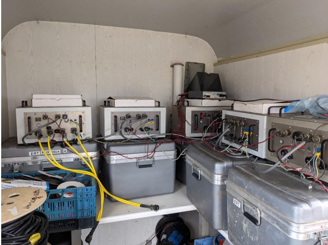
Figure 3 The main measuring unit with the extension switch boxes.
