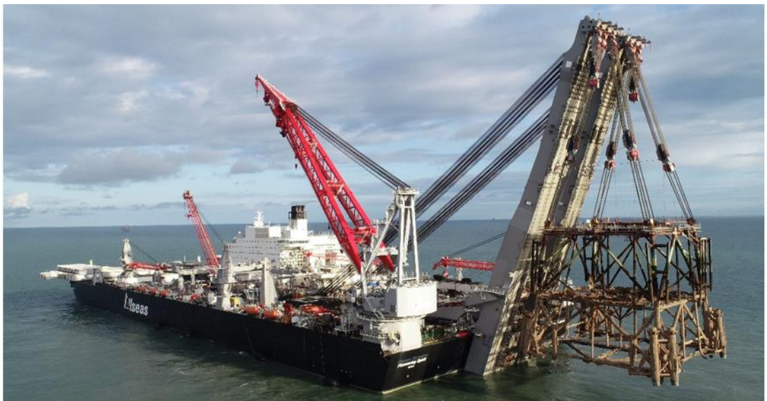
Figure 6.4 Allseas Morecambe project. The Pioneering Spirit lifting the first offshore jacket. Operations are timed favourably (during slack water) by means of the TKI Ocean Race Pilot.
