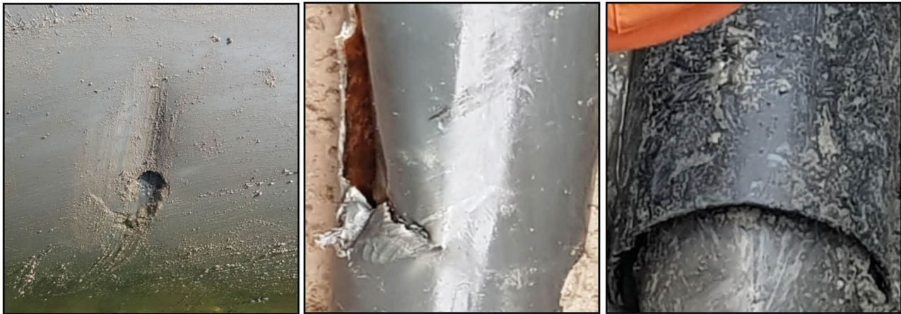
Figure 9. In-situ footage after excavation of pipes A-3 (left) and B-2 (middle) with break due to third party impact, and pipe B-3 (right) with crack due to poor installation quality.
