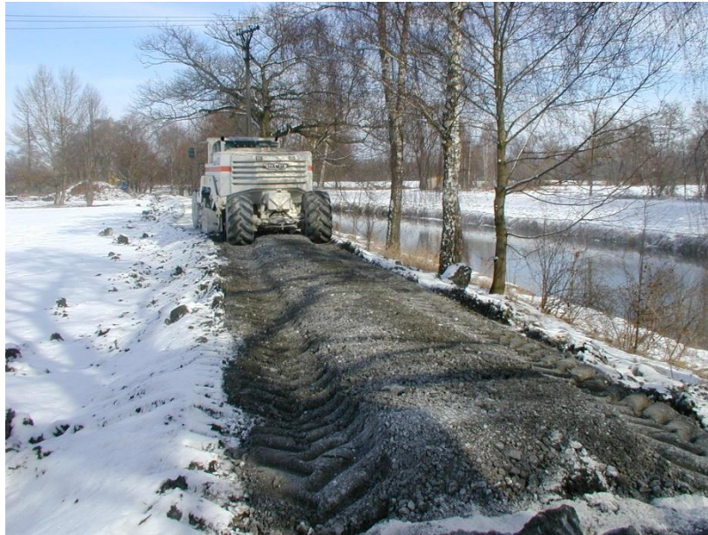
Figure 3.7. Soil treatment technology with Proviacal ® used during building of flood dike in Hradec Králové.
