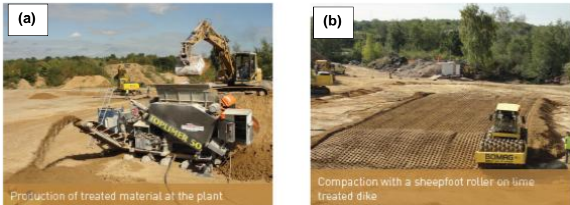
Figure 3.2 (a) Production of treated material at the plant and (b) compaction with a sheepfoot roller on lime treated dike.
