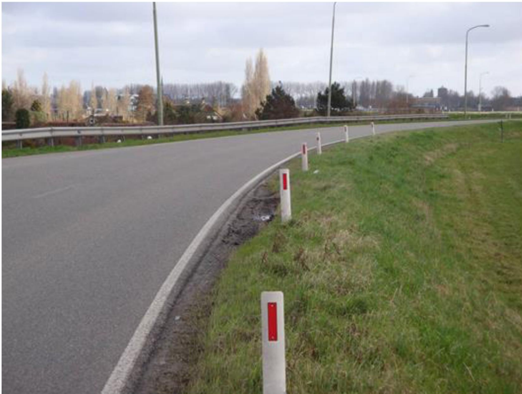
Figuur 5.2. Transition from the road to the grass cover is a weak point
