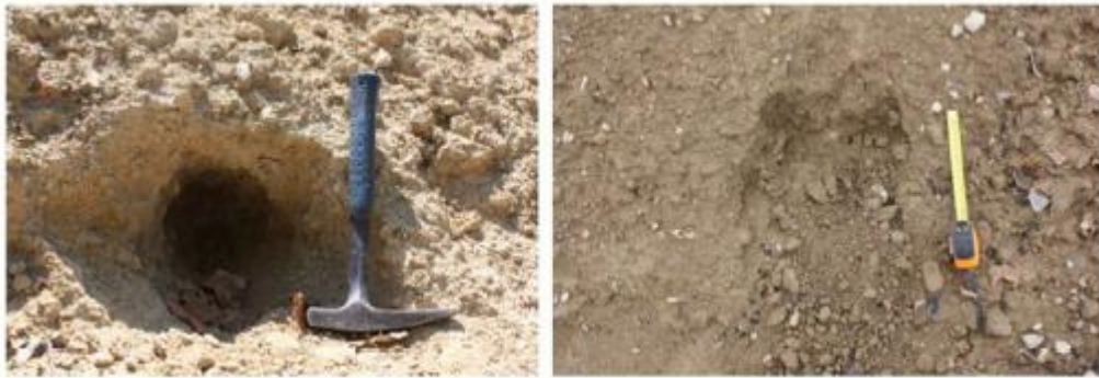
Figuur 4.1. Burrowing animals holes in non - treated soil (left) and unsuccessful attempts in lime treated soil (right). (after Nerincx et al. 2016).
