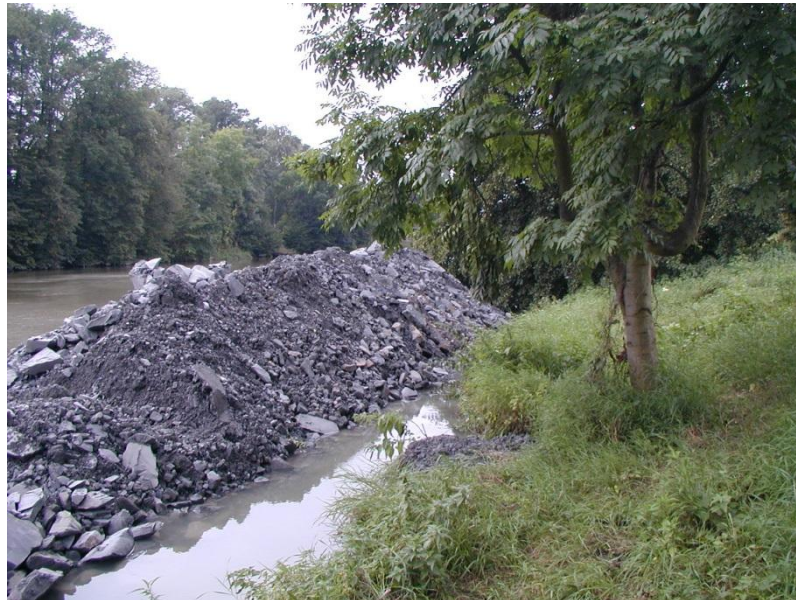
Figure 3.8. Excavated sediment from Labe river near Pardubice is treated with Proviacal ® and used for flood dikes construction.
