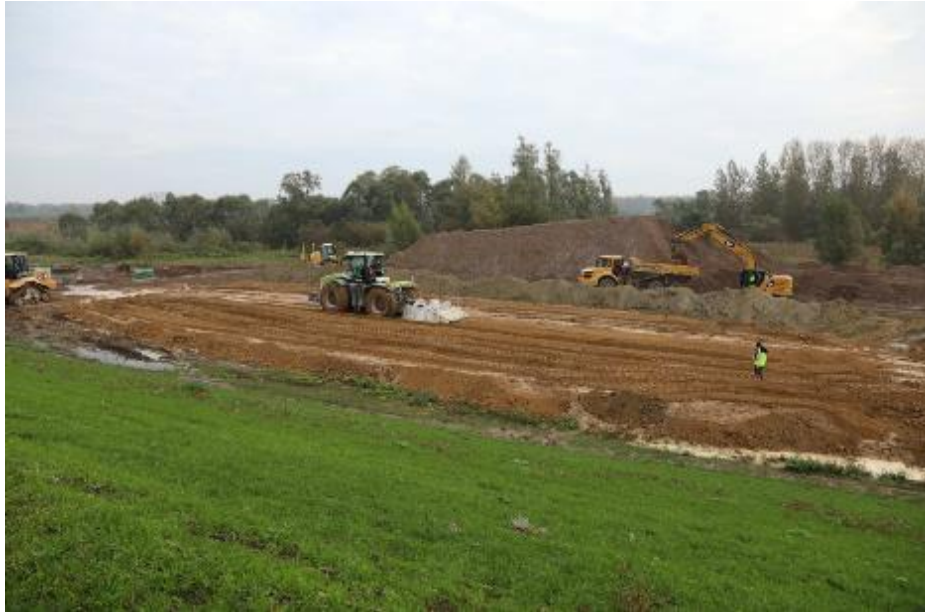
Figure 3-3 View of production platform at Vlassenbroek polder.
