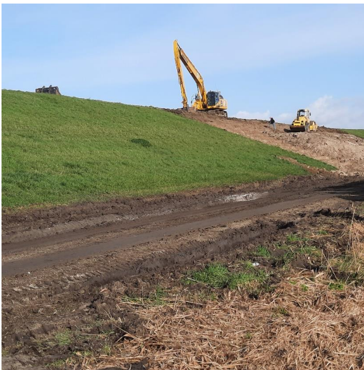
Figure 3-11 Long armed excavator crane and compactor on the slope of the dike.
