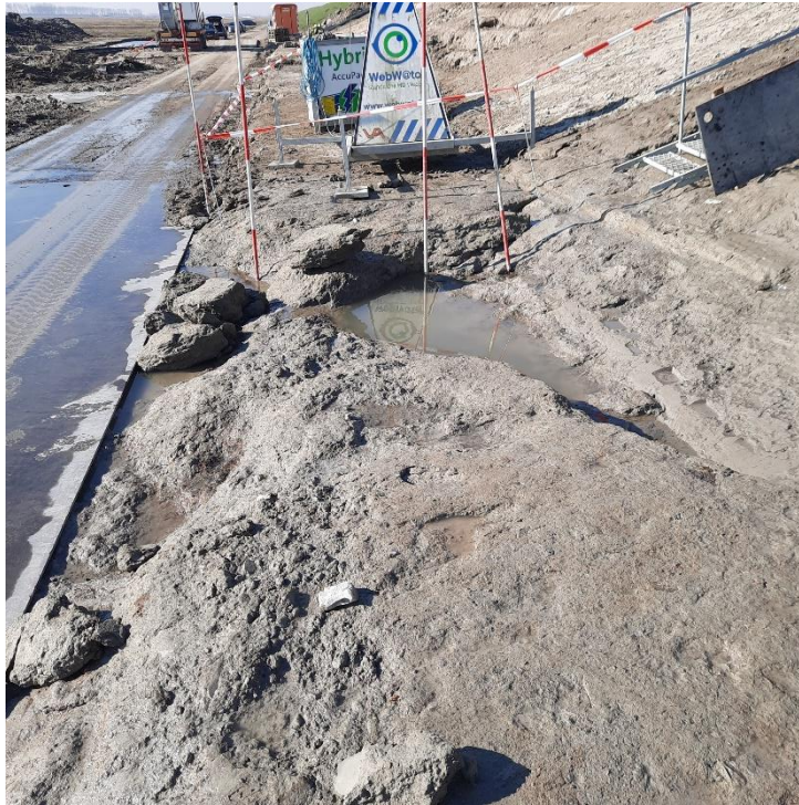
Figure 8-13 Erosion on the berm in section 2B.
