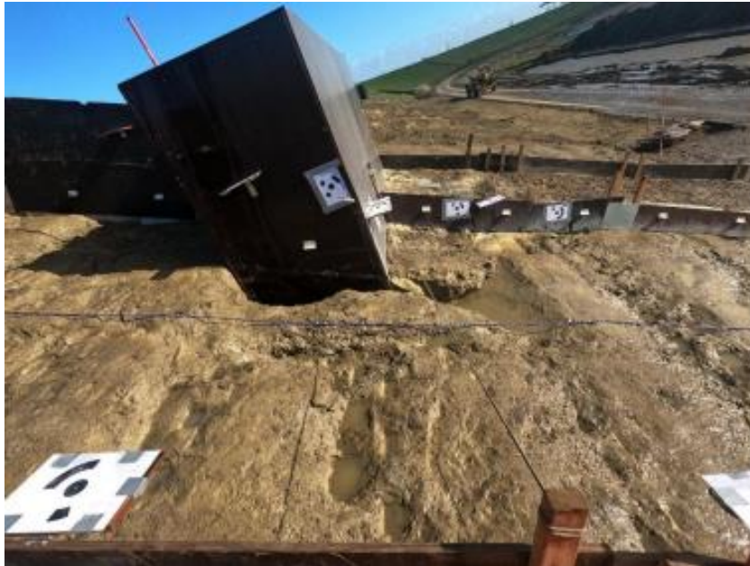
Figure 6-3 Erosion also below the obstacle.
