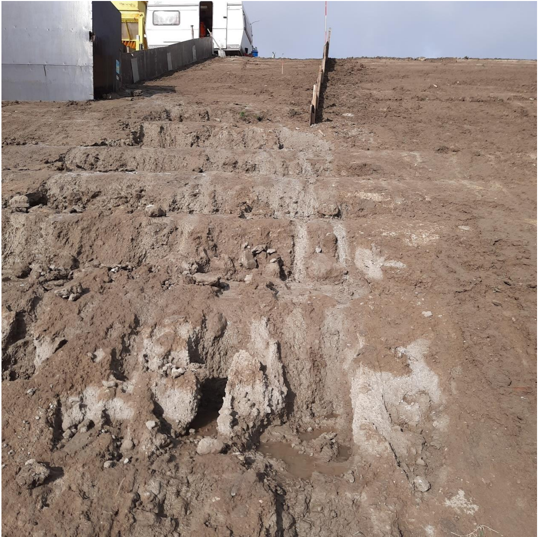
Figure 8-12 Erosion in the lower part of Section 2B.
