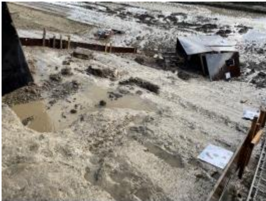
Figure 6-4 The failed obstacle.
