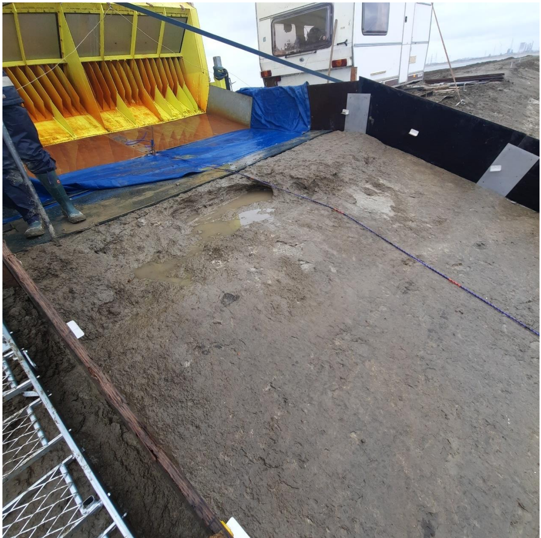
Figure 8-11 Erosion near the crest in section 1A.
