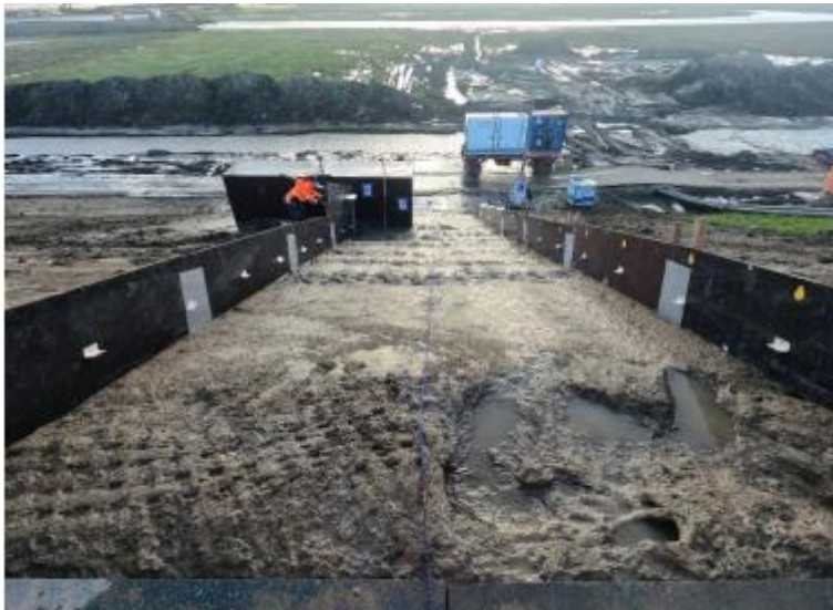
Figure 6-2 Erosion near the crest after 50 l/s/m'.
