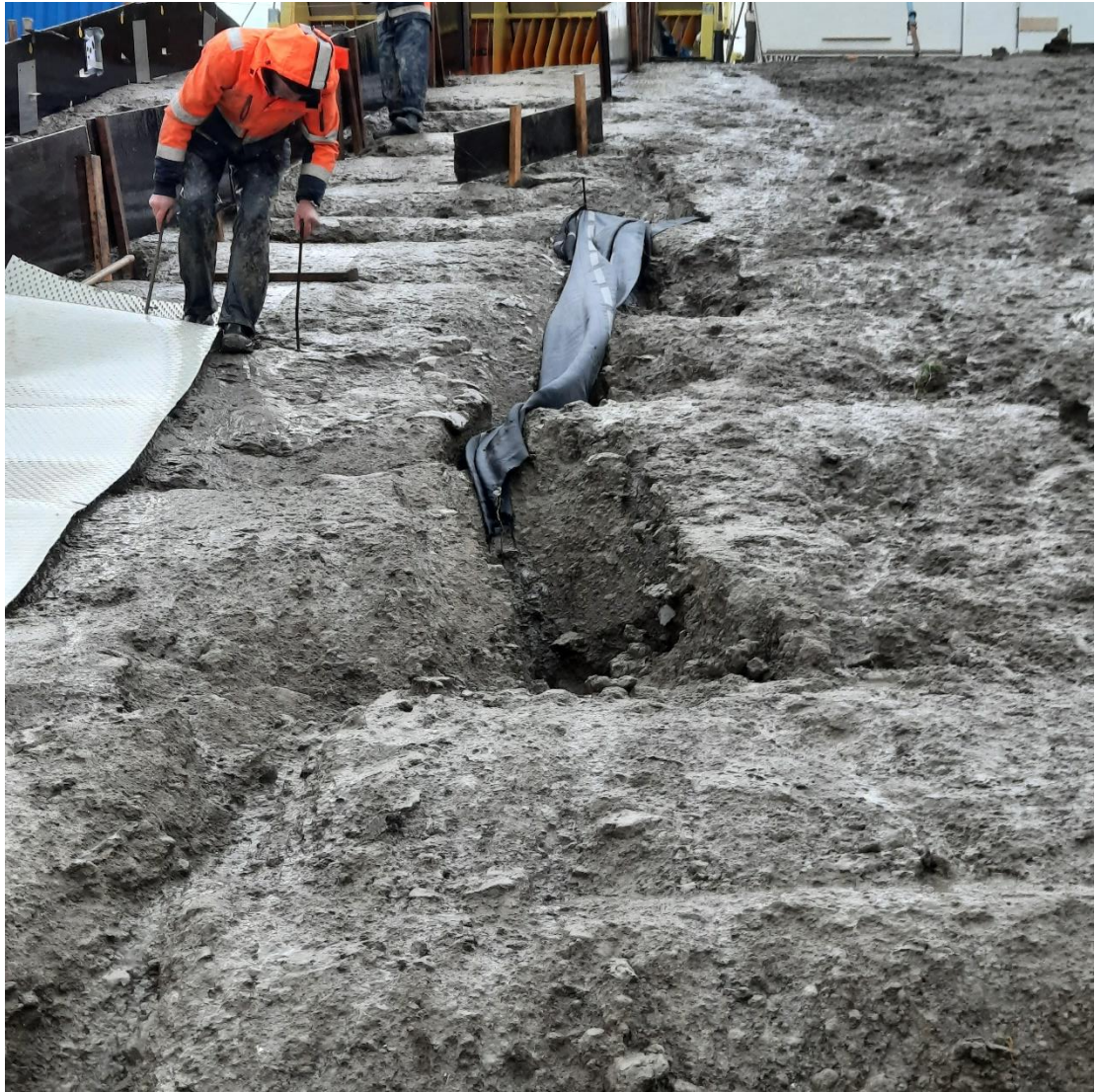
Figure 8-14 The difference between compacted treated clay and non compacted treated clay: the large erosion gaps are on the boundary between treated and densified material and material from the transition zone where no compaction took place. The erosion gullies are not the result of very large amounts of water flowing down the slope, but result from leakage water underneath the boarding of the test section.
