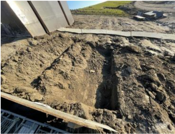
Figure 6-11 A Vertical cliff was dug into the slope (picture courtesy of Infram).
