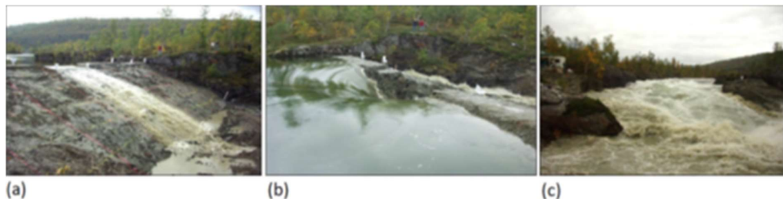
Figure 5: Impression of the complicated hydrodynamic conditions during breach formation
