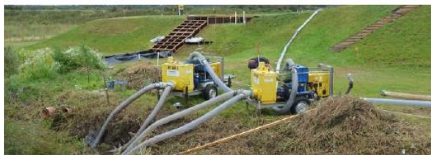
Figure All.13. Two pumps deliver water into the polders
