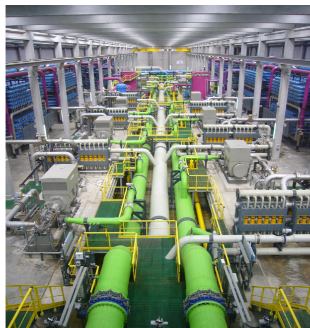
Figure 4: Pipe networks inside a RO plant (image: James Grellier).
