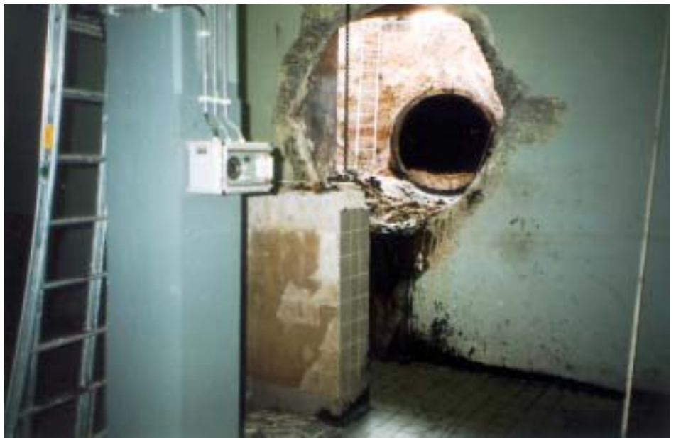
Unanticipated fluid transients may cause severe damage
