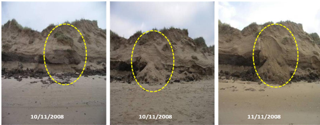
Dune toe erosion: National Trust car park, Formby Point
