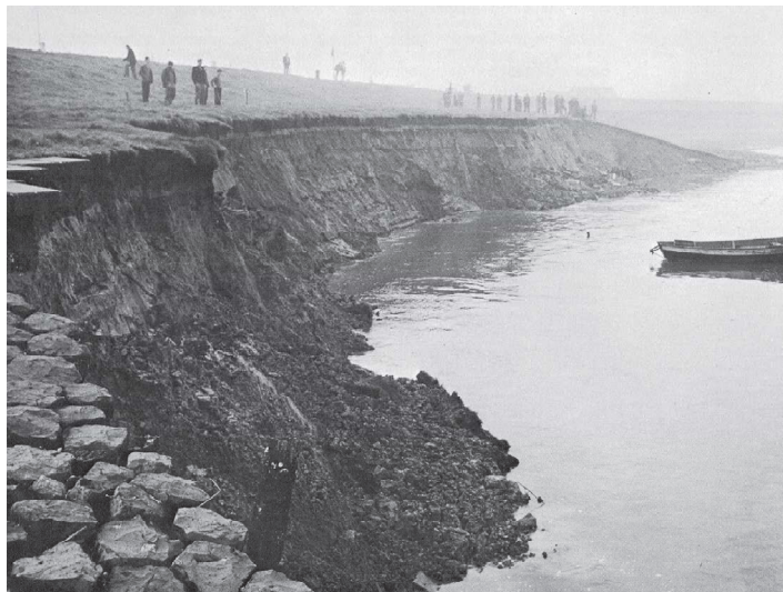
Figure 2.1-1: Slope failure which resulted in damage to a dyke.
